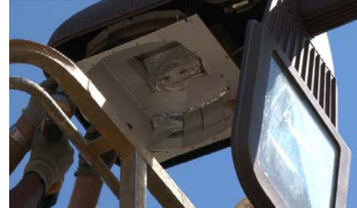
FIGURE 1: Opening cover for parking lot fixture to remove reflector and electrical components
