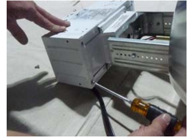
FIGURE 1: Unscrewing the outer plate of the enclosure.
