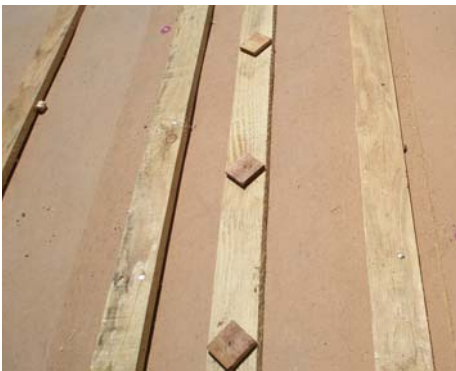
Raised batten installed with one piece turned over to show blocks preattached
