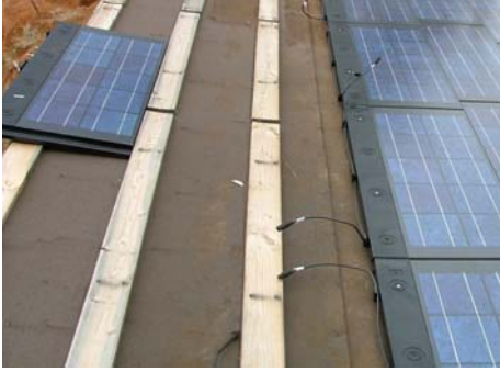
Battens fastened to deck, no air space
